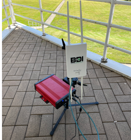
Figure 6.1.1: Wireless Base Station mounted on tripod with Router
