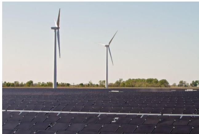
Figure 4: Solar and wind farm in Woodstock, Minnesota [4]
