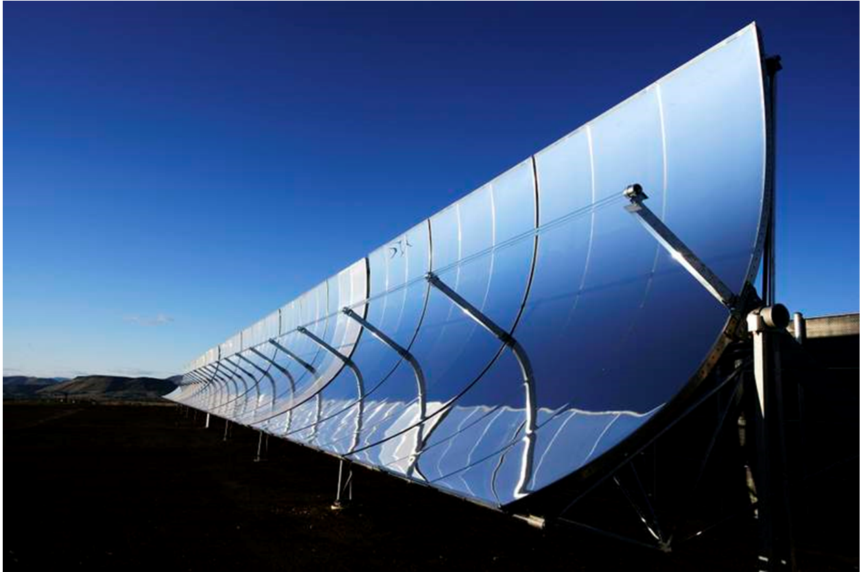
Figure 7: An example of a parabolic trough CSP system [10]
