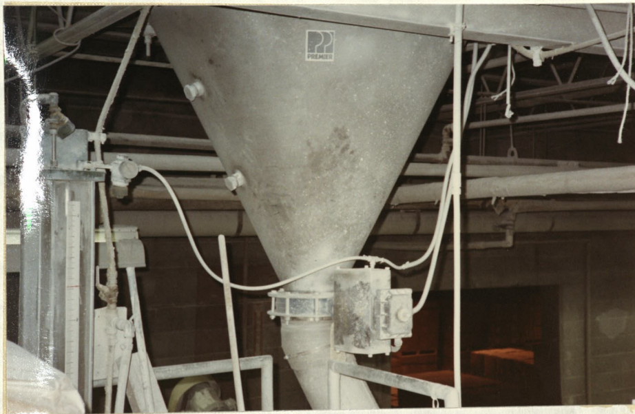
Figure 9. PVC Resin Hopper.
