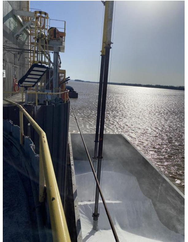
Figure 20: Alumina Unloading System
