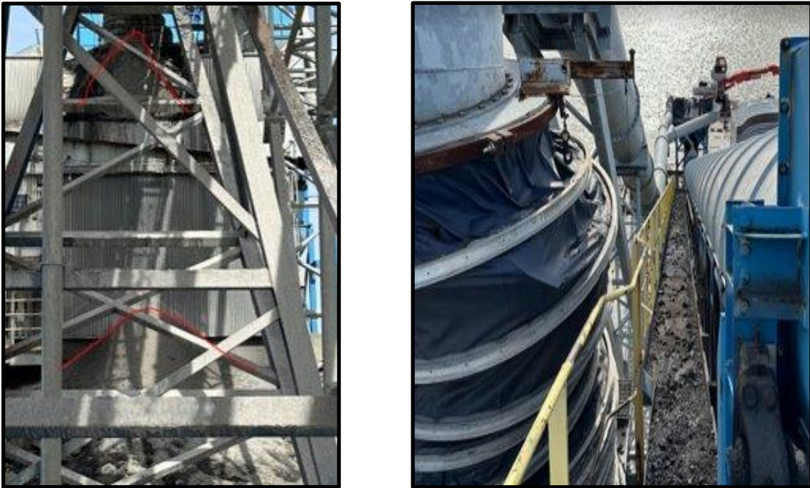
Figure 11: Material Build Up on Current System
