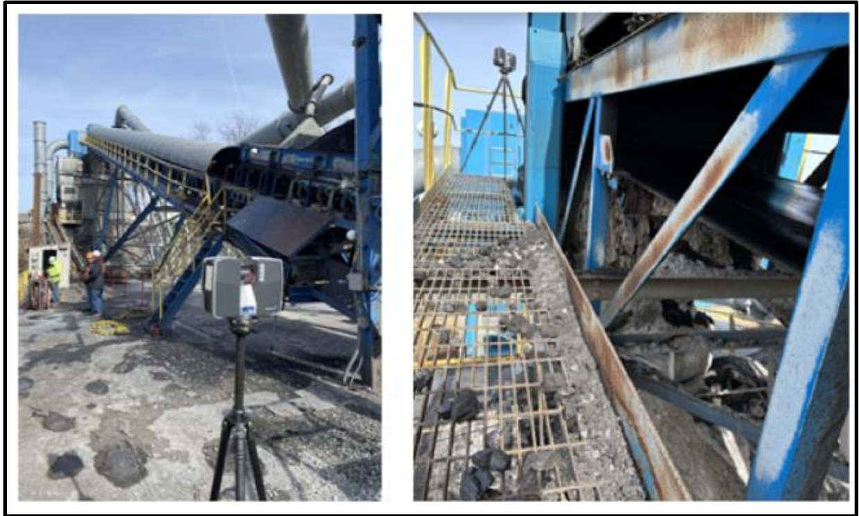
Figure 4: Current Conveyor on Dock Barge at Alcoa (Owned by EMS)
