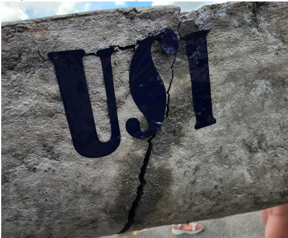
Figure 21. Crack in the End Cap on Race Day.
