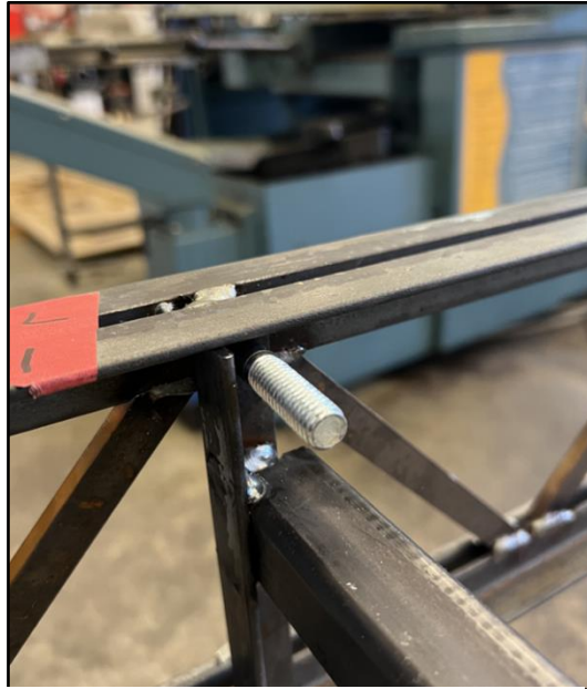
Figure 41. Lateral System Issues
