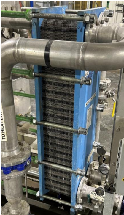
Figure 1: Funky Plate and Frame Heat Exchanger
