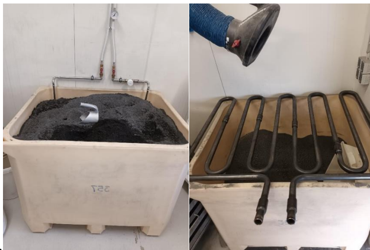
Figure 14. Current Sand Dryer at the Blue Lagoon
