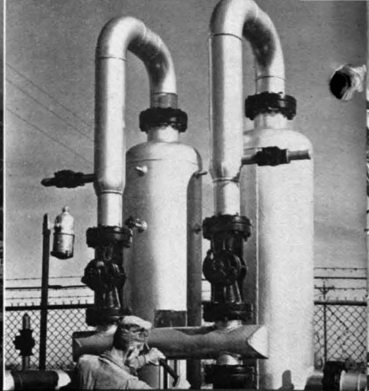
Propane gas stand-by plant. In rear, propane storage tanks, capacity 300,000 gallons.
