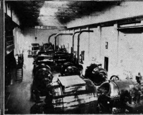
TURBINE ROOM - DIVISION ST. STATION
