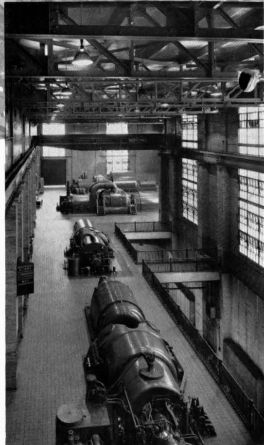
Turbine-generator room at Ohio River station, showing four of the five present units.
