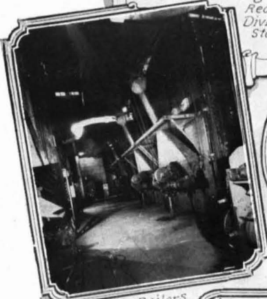
2 New 512 H.P. Boilers Division St. Station
