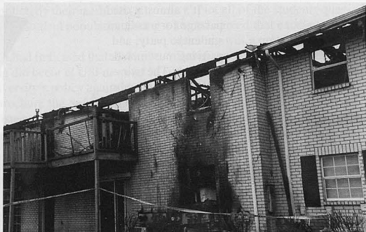
Below: Student housing located at Shiloh Place, off Covert Ave., was severely damaged by fire.
