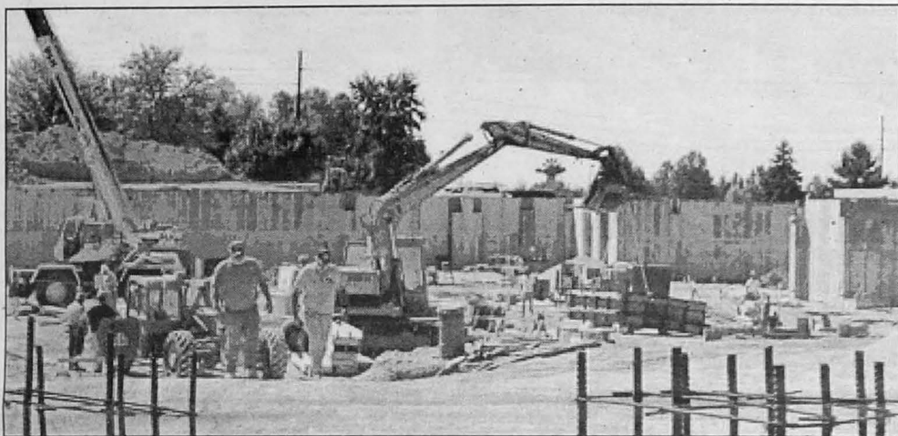
Construction crews work on the new library foundation Tuesday. The foundation walls are more than half-way finished. The library is set to open summer of 2006 (photo by Randy Hawkins).
