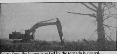
Debris from the homes wrecked by the tornado is cleared. Photo by Julia Hunter
