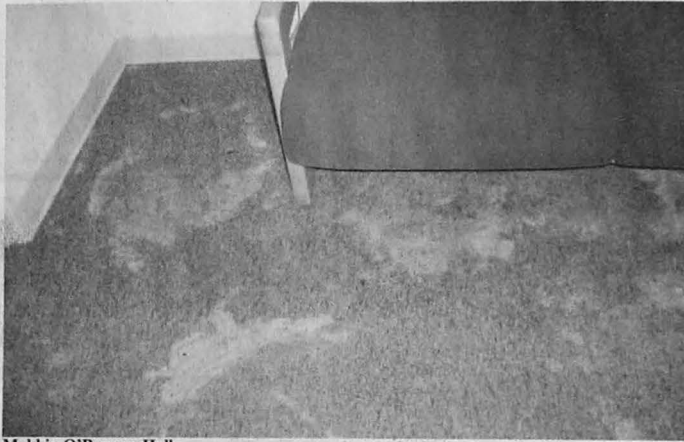
Mold in O'Bannon Hall.
