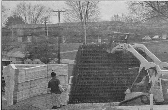
USI campus housing can be seen across Schutte Road from the construction site of the new Eagle Village apartment complex. The new apartments are set to open in time for the 2005 fall semester (photo by Randy Hawkins).
