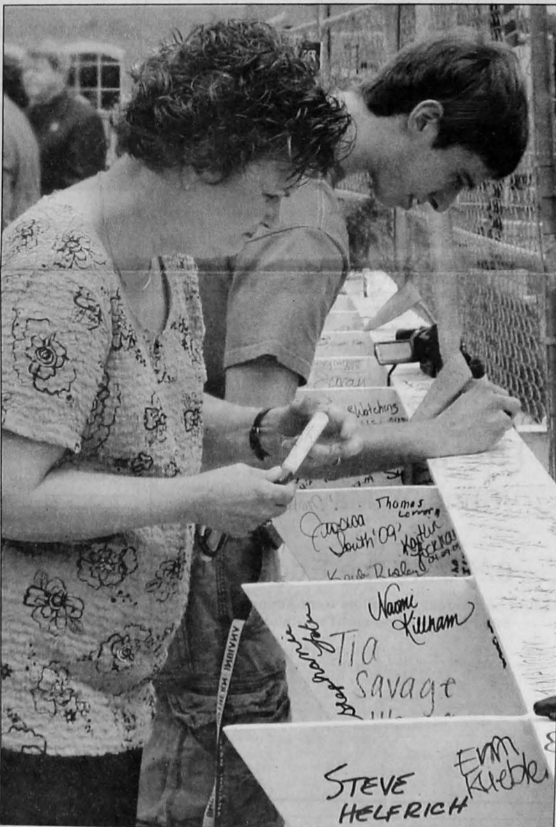
USI student Logan Storrer and Chris Jines of career services sign the final beam of the Business and Engineering Center to be put in place. Members of the campus community signed the beam throughout the week in anticipation for last Thursday's topping off ceremony. The day's celebrations also included the groundbreaking for the University Center expansion, which will include a new UC bridge and a newly constructed tower.
