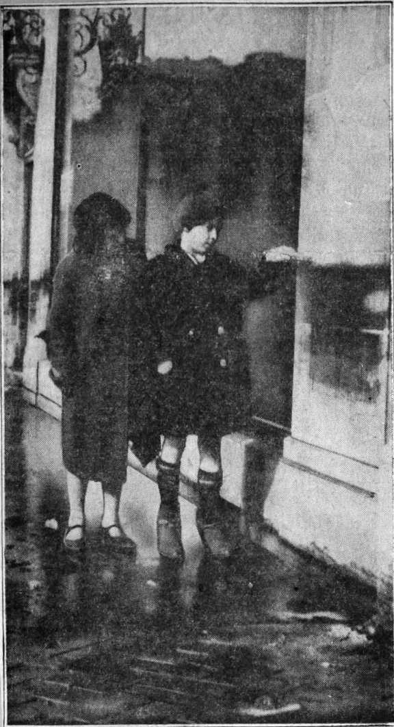
HEIGHT REACHED BY FLOOD WATERS — Two Louisville, Ky., children indicating the line on downtown building which was made by the dirty waters of the Ohio. The river was dropping rapidly at Louisville yesterday as the city started on the task of rehabilitation.
